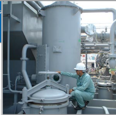
Above: Scrubber for Aalborg Industries™ flue gas type inert gas system.
